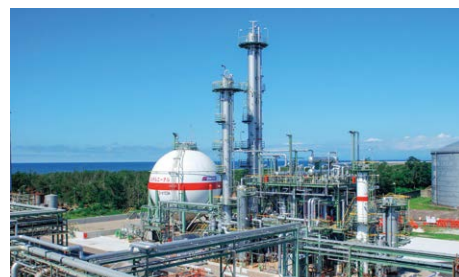
Our DME plant at the Niigata Plant
