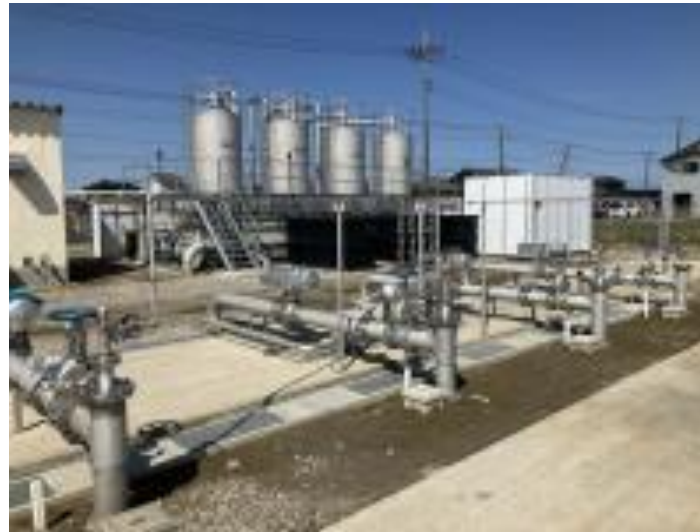
Water-dissolved natural gas production facility
