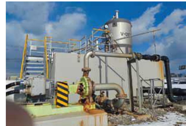
Current water-dissolved natural gas production facility
