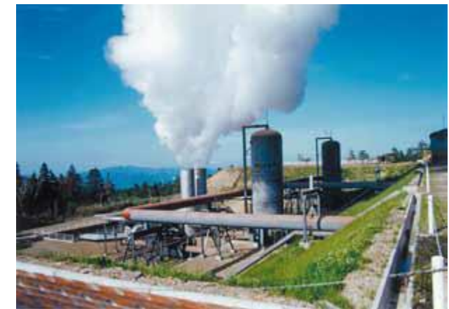
Steam releasing at Sumikawa Geothermal Power Station
