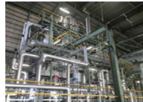
Methanol pilot facility (Niigata Plant)
