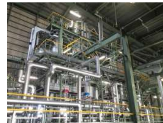
Methanol pilot facility at Niigata Plant
