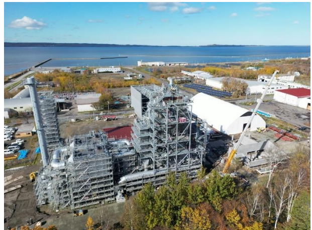
(3rd power plant)
